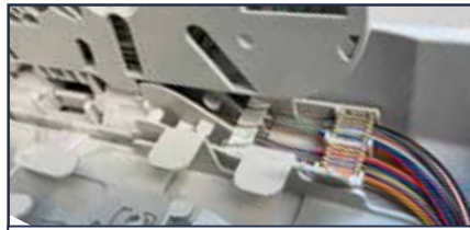
Pigtails well arranged to splice cassettes with intuitively designed bridges
