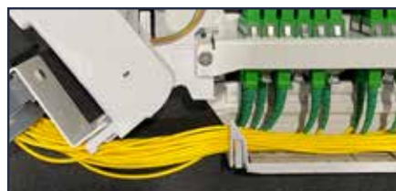
Patchcords guided to the side, protected by front door with label for port identification
